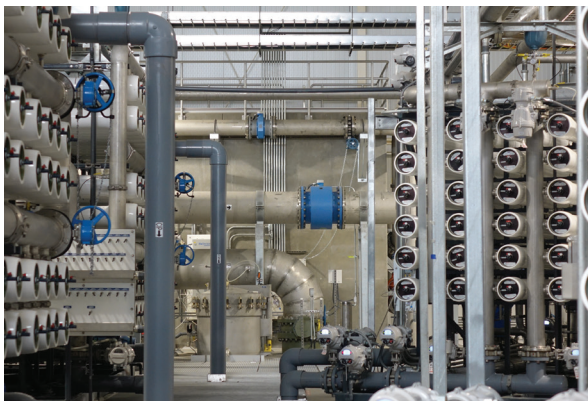
A portion of the reverse osmosis filtration system inside the ECCV Northern Water Treatment Plant. The plant converts renewable water from the South Platte River into faucet-ready drinking water for ECCV customers.
